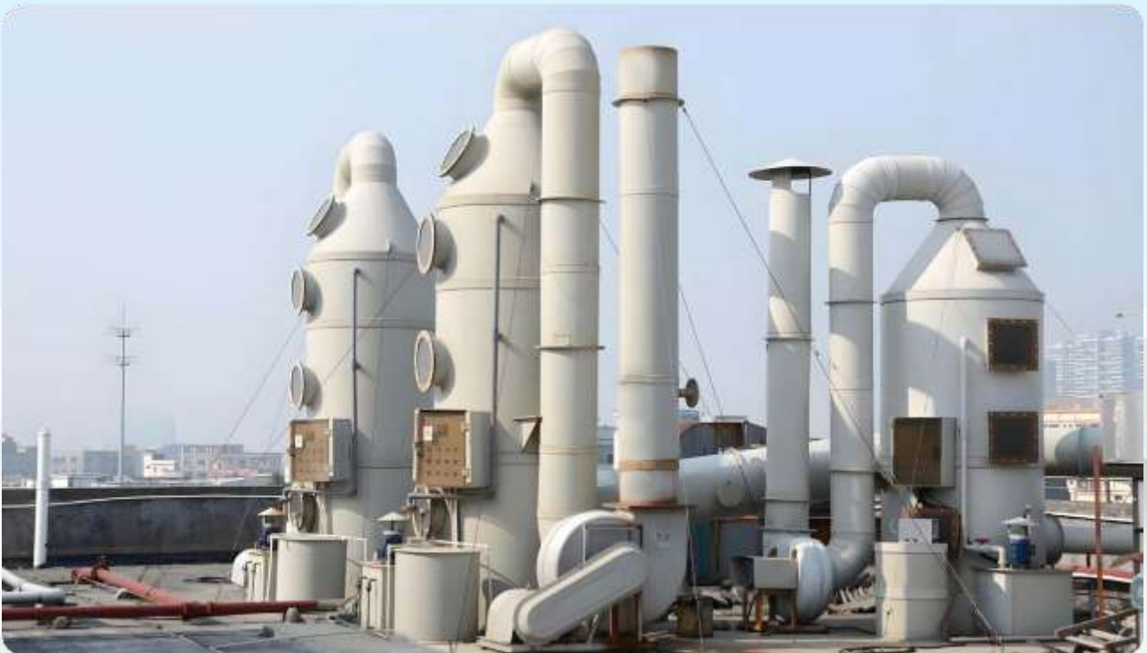
■ 安阳瑞美达清洁能源废气处理设备安装项目 Anyang Ruimeida Clean Energy Waste Gas Treatment Equipment Installation Project
