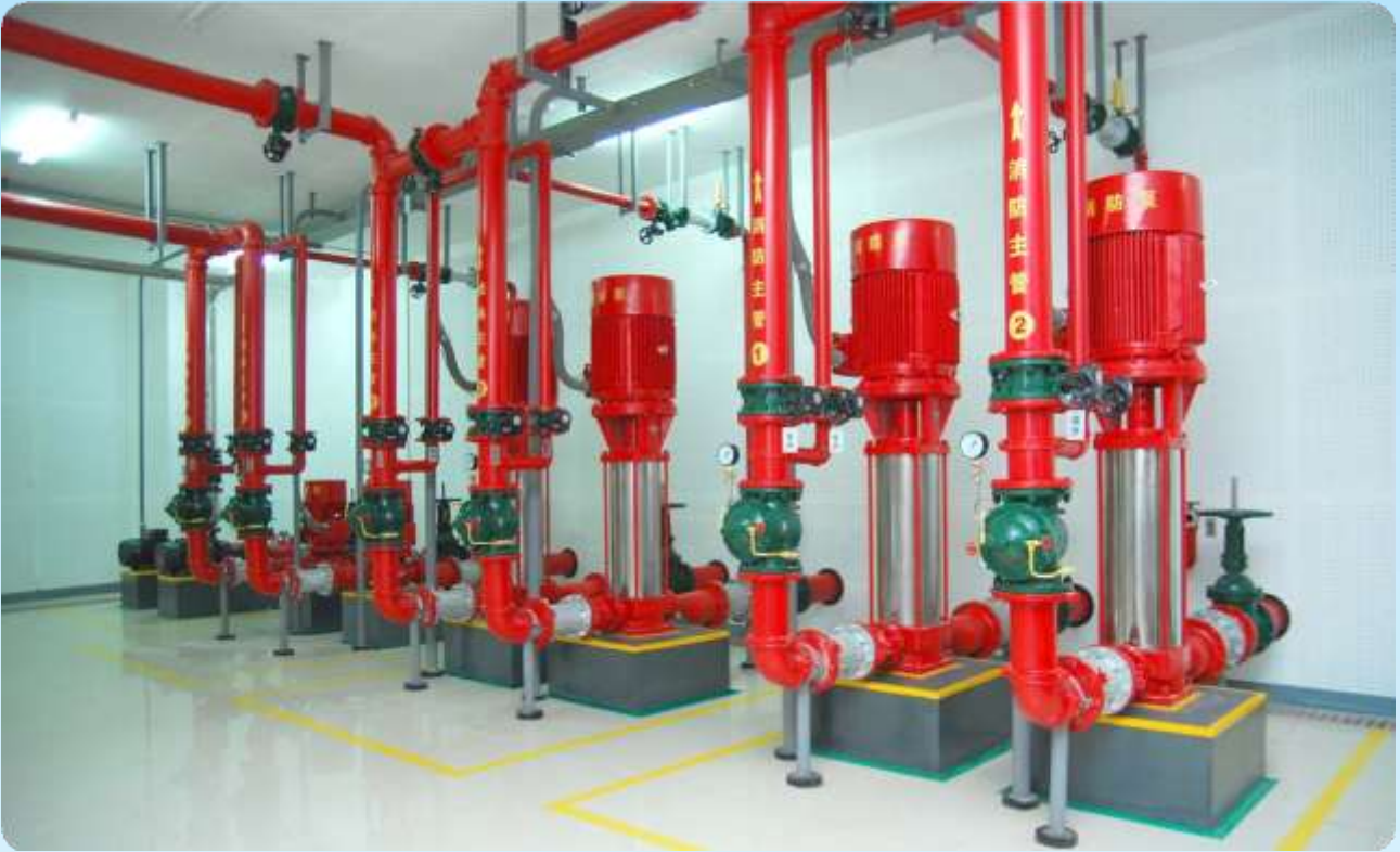
■ 领秀城消防设施安装项目 / Lingxiu City Fire Protection Facility Installation Project
