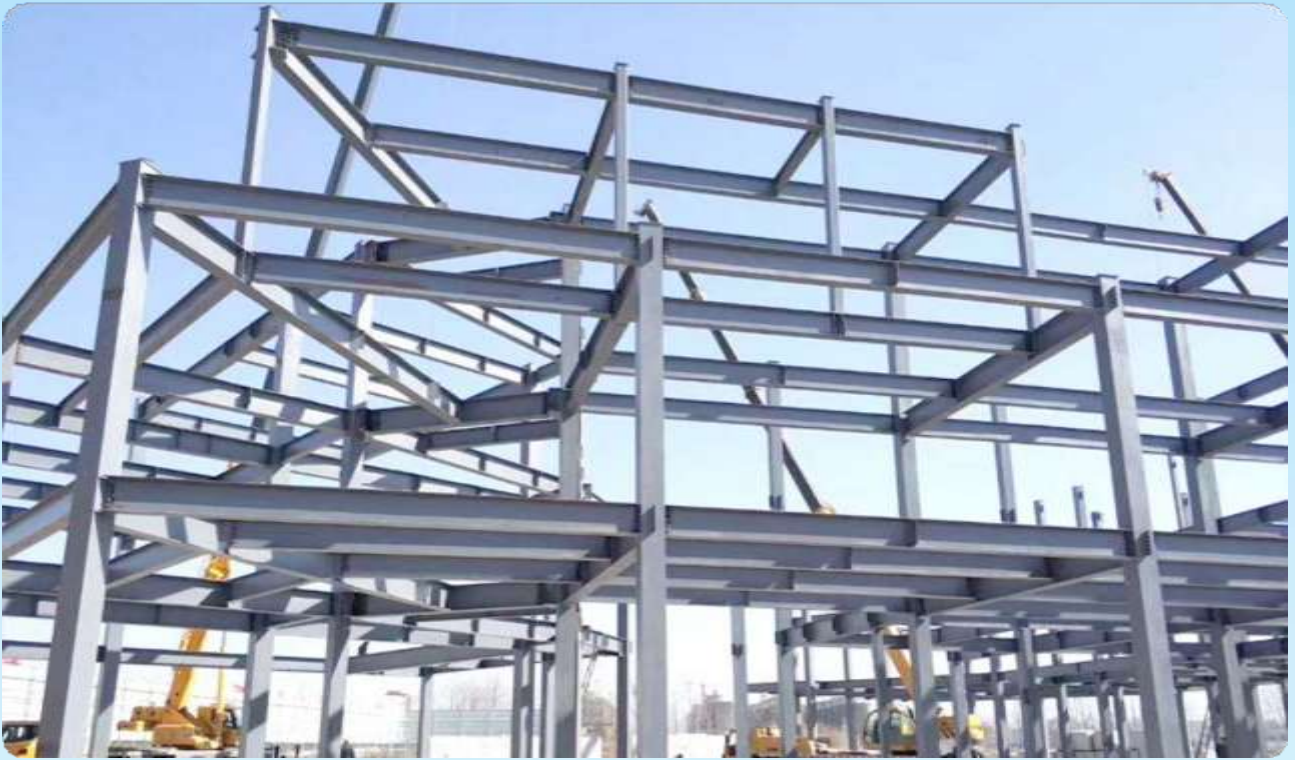
■ 牧原农牧猪舍土建及附属工程/ Construction And Ancillary Works Of Muyuan Agricultural And Livestock Pig House
