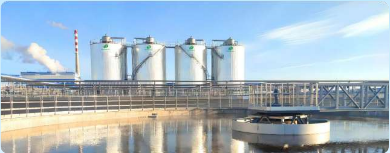
■ 兰州市污水处理厂升级改造项目 / Lanzhou Sewage Treatment Plant Upgrade And Renovation Project
