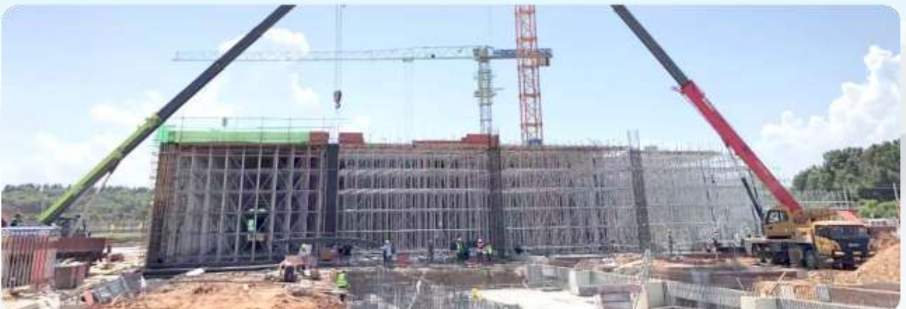
■ 湖北吉利硅谷初洗车间附属楼/Hubei Geely Silicon Valley Primary Cleaning Workshop Annex Building
