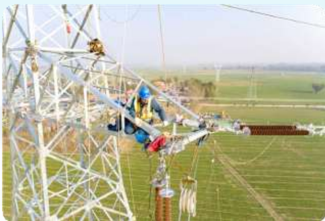
35kV 高河高压线路升级改造 35kV Gaohe High Voltage Line Upgrade And Renovation
